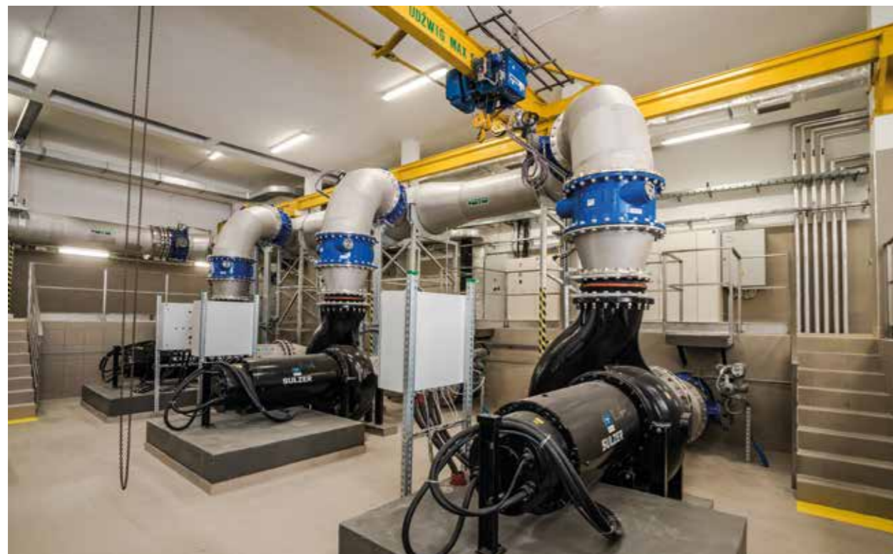
Nowoczesne pompy SUW „Filtry” / Pumps in “Filtry” water treatment station Fot. Krzysztof Kobus/Travelphoto.pl
